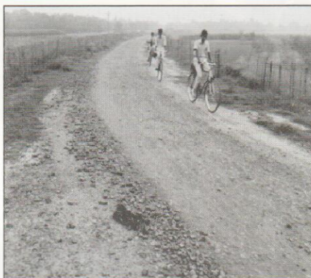
Figure A : Damaged Road
